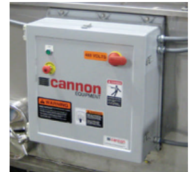
Main Control Box
